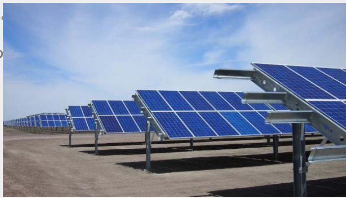
Stillwater Solar-Geothermal Hybrid project. Image courtesy of the Nevada State Office of Energy.
