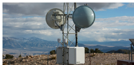
The cyberinfrastructure data transport network allows field scientists to make connections between equipment, database systems, the internet, and each other. --Scotty Strachan Photo
